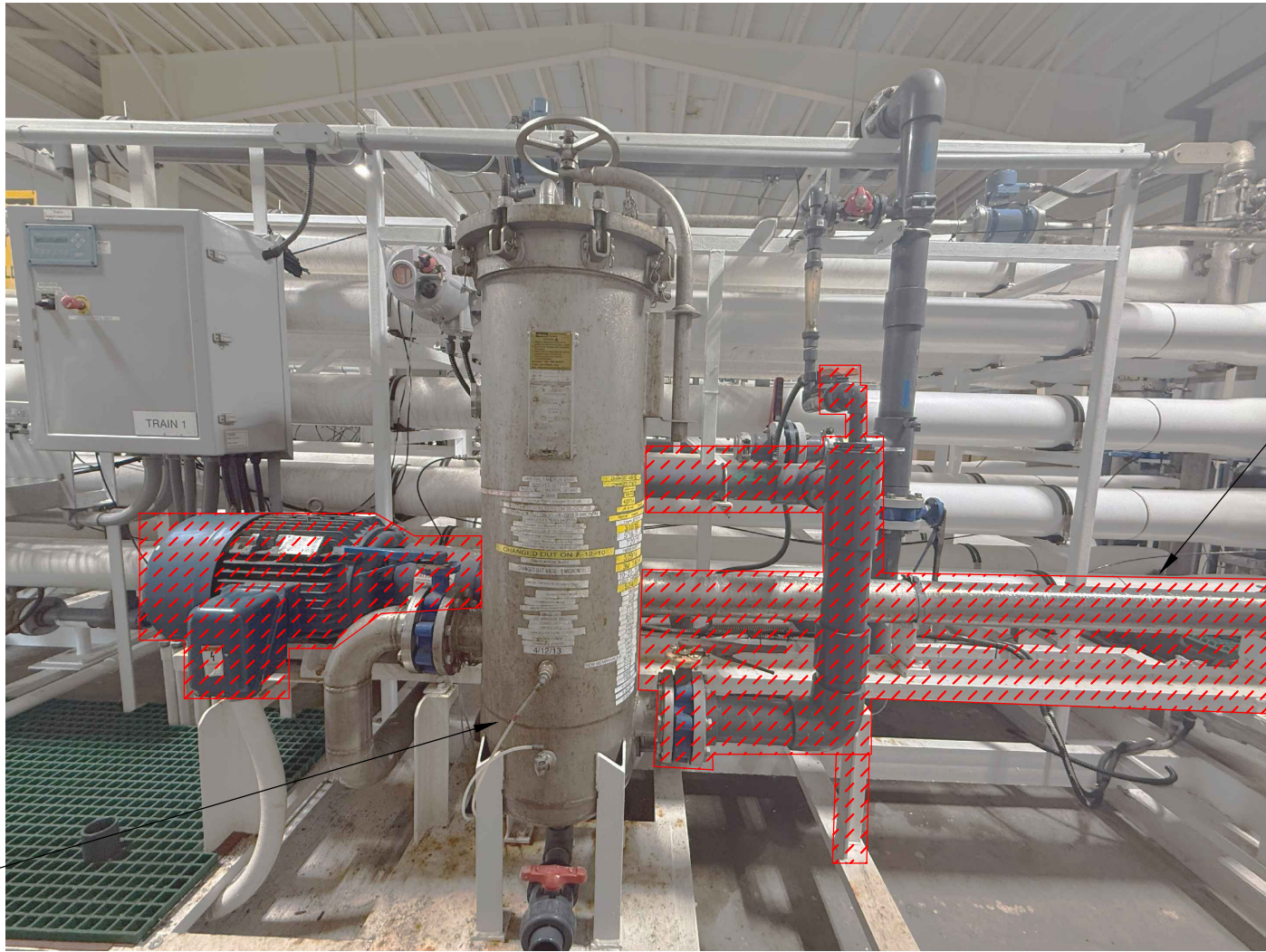
TYPICAL EXISTING RO SKID FEED PUMP, MOTOR, BASE AND SUCTION PIPING PHOTOGRAPH 4 NTS
