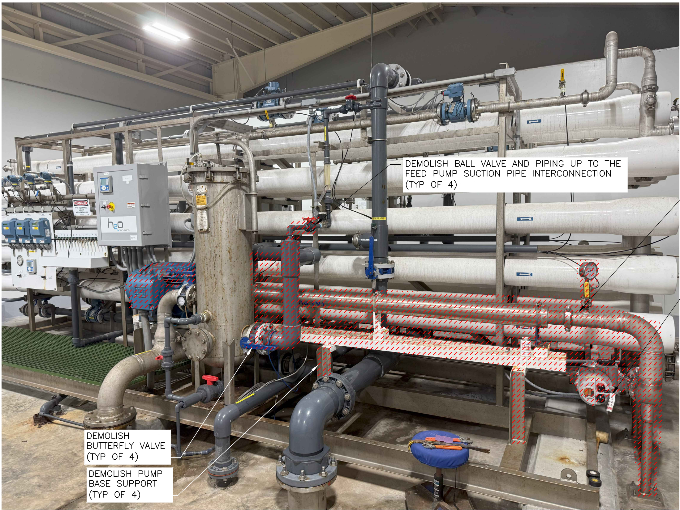
TYPICAL EXISTING RO SKID FEED PUMP-SIDE PROFILE PHOTOGRAPH 1 NTS
