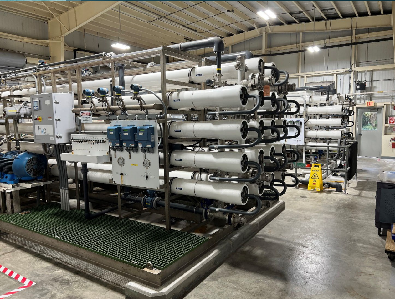
Reverse Osmosis Membranes
