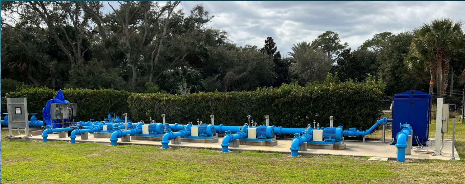
Water Distribution Pumps
