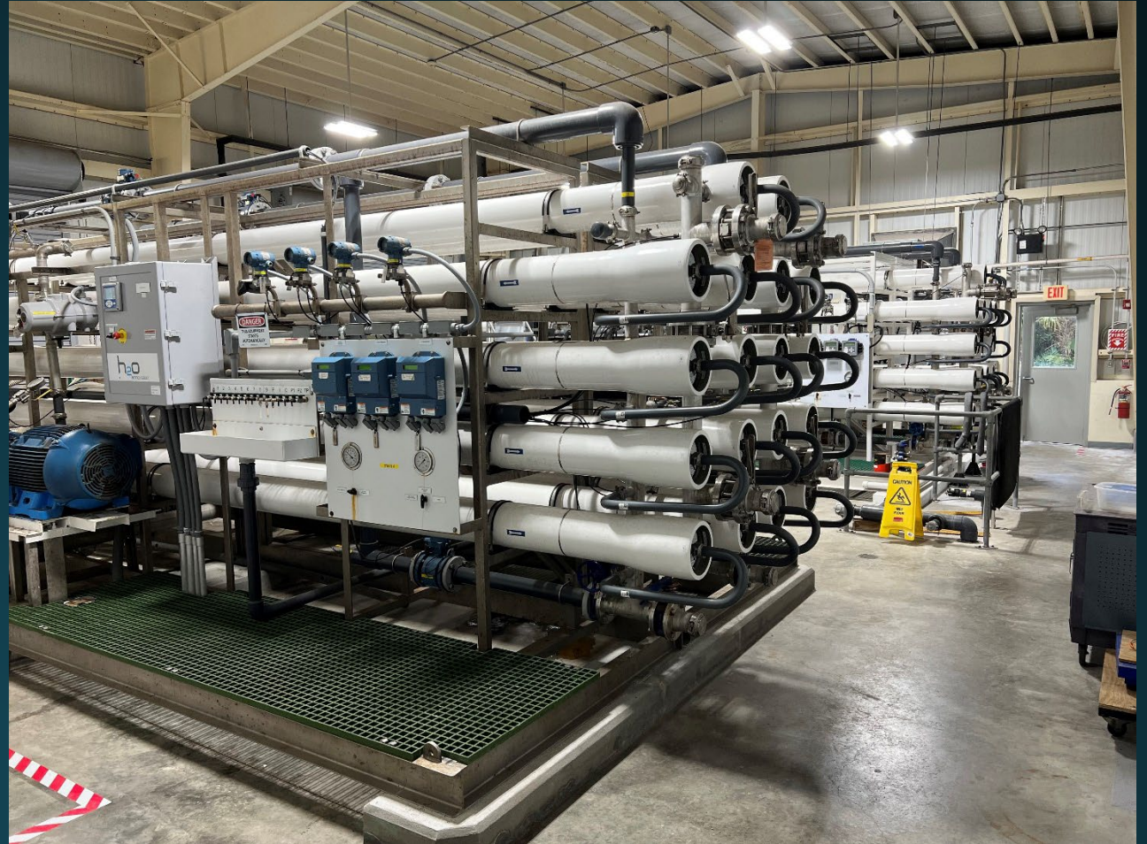
Reverse Osmosis Membranes
